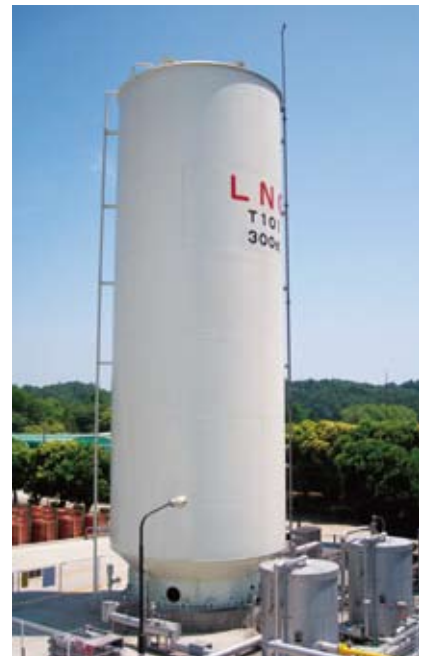
LNG storage facility (Toyouura Works)
