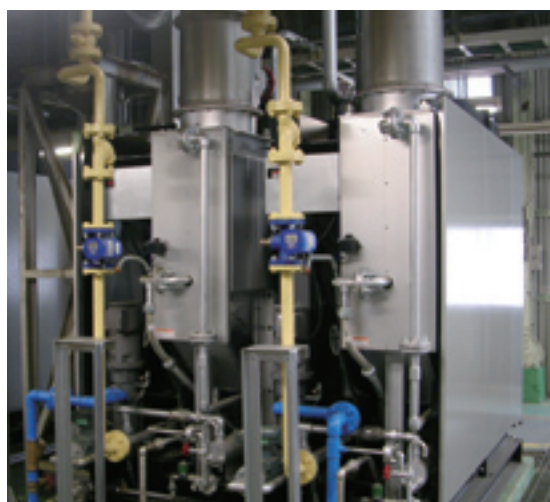
City gas boiler (Densen Works)
